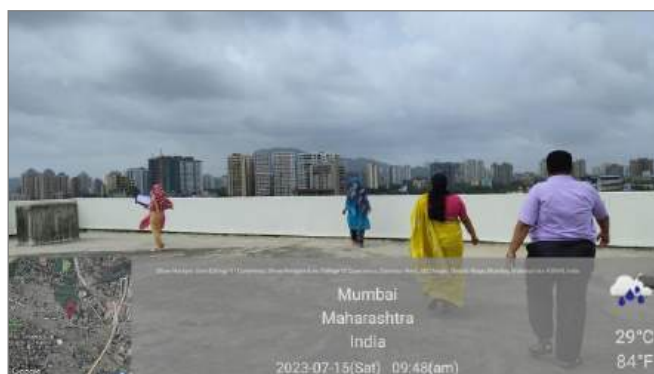
Investigative parameters – Site Aspects – Terrace study to understand waterproofing and cooling study
