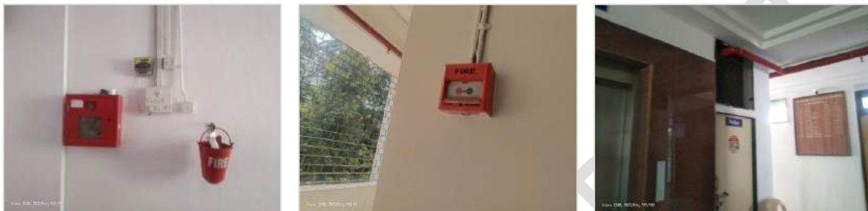
Plate 4: Fire and life safety measures undertaken
